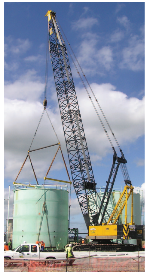
A large crane is used to shift the empty acid storage tanks to concrete foundation pads
