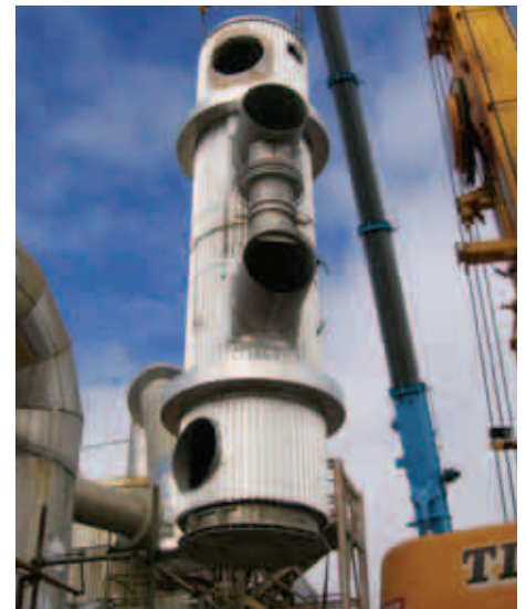
The hot heat exchanger moves into place
